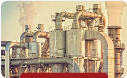
Acid gas enrichment in gas processing unit
